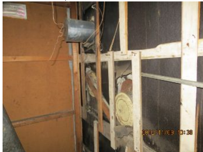
unsecured holes in exterior walls is observed. Should have been repaired.
