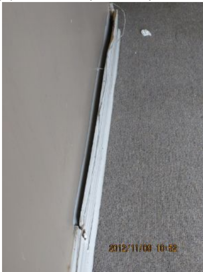
Damage(s) noted. required repair and painting.
