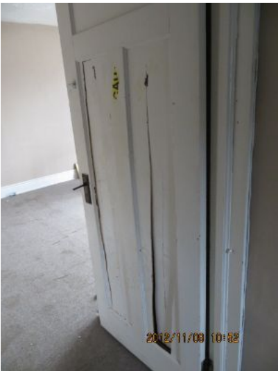
Some or most doors were broken. Required replacing.
