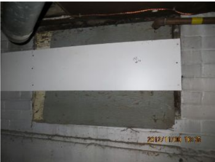
Some or all windows were blocked with materials or storage. Has to be open.
