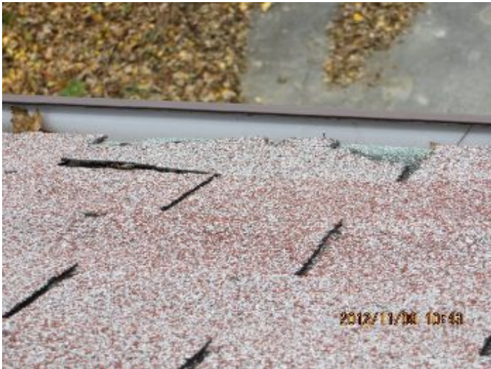
Lifting at laps and around roof vents observed.
