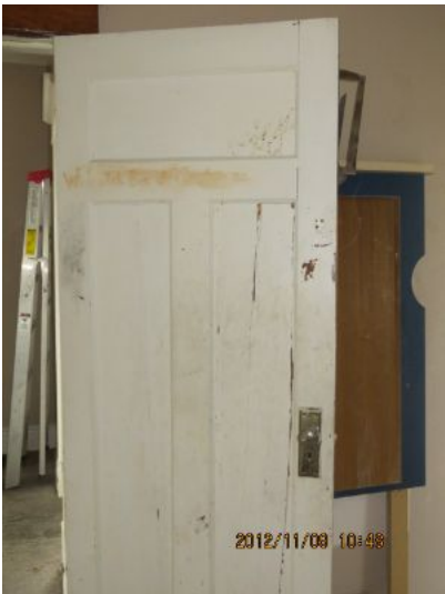
Damage(s) noted. required repair and painting.
