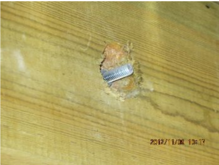
Deck appears to be nailed to the structure or anchor bolt has been used into veneer, which is not meet today building code, through out Bolts secured to the house framing are required by most municipalities. We recommend reviewing local standards for safety and compliance. further check is required.
