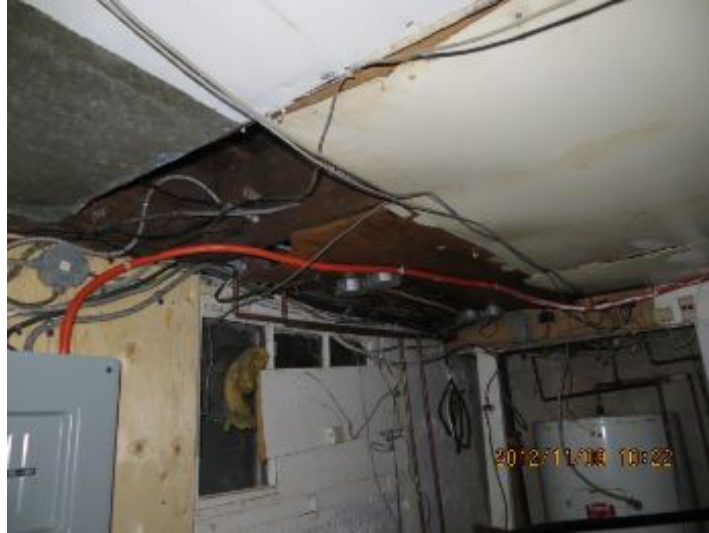
Ceiling is sagging.
