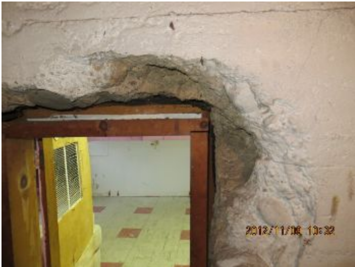
Foundation wall(s) have been cut or bored. The foundation wall is not structurally supported. Instalation proper lintel is required.
