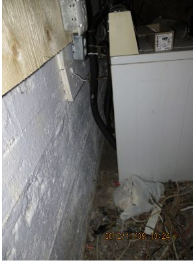
Dryer is not hooked up
