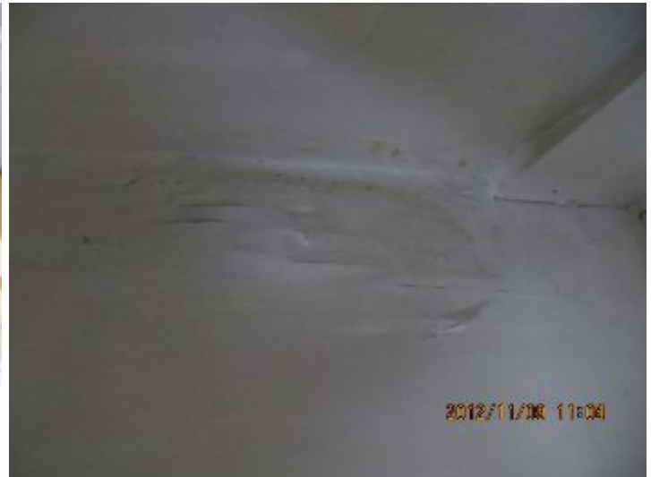
Evidence of past water penetration observed. At:
