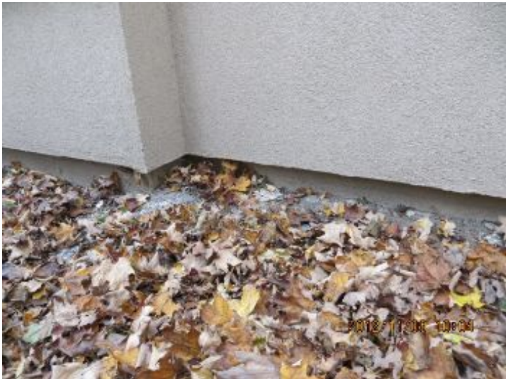
inaccessible (covered by material)At: all around
