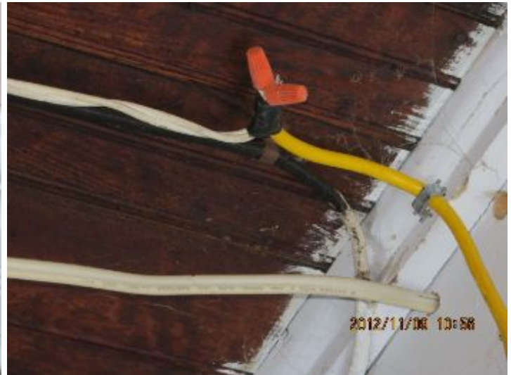
Improper use of extension cord observed. Extension cords should not be permanently installed or be routed through walls, floors or partitions.
