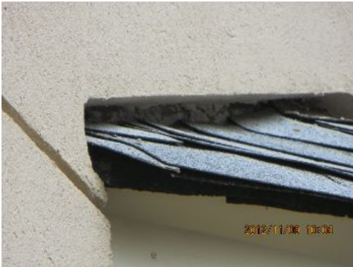
Missing counter flashing. Installation proper counter flashing recommended.
