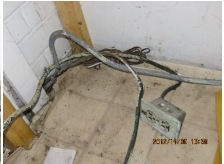
Exposed wires observed. Recommend review by a licensed electrician for repair or replacement, as necessary, prior to close.
