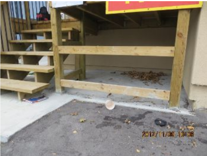
Improper installation of column to pilar, lack of proper bracket or hanger was appeared. This situation is structure not supported, installation proper bracket to improve deck structure is required.
