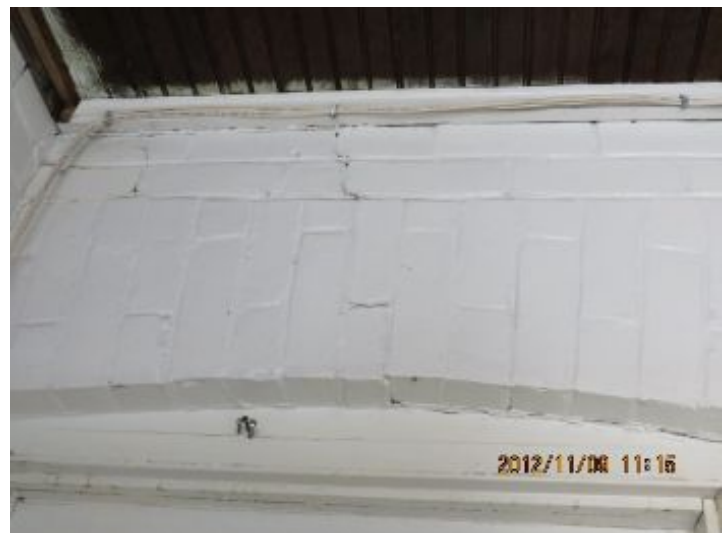
Settlement crack(s) observed. At: rear, extension part.
