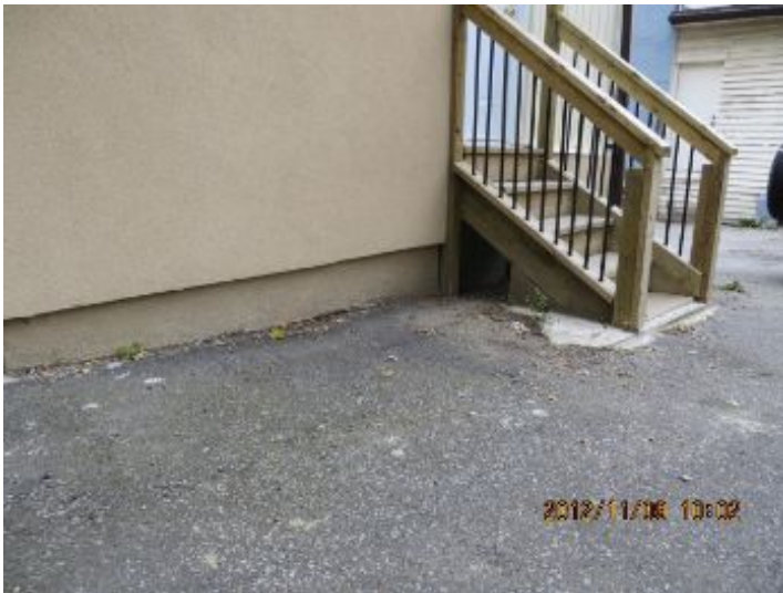
Grading slopes toward the foundation walls. Correction/improvement is needed. at: rear and east
