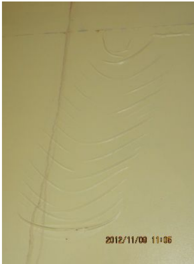
Evidence of past water penetration observed.
