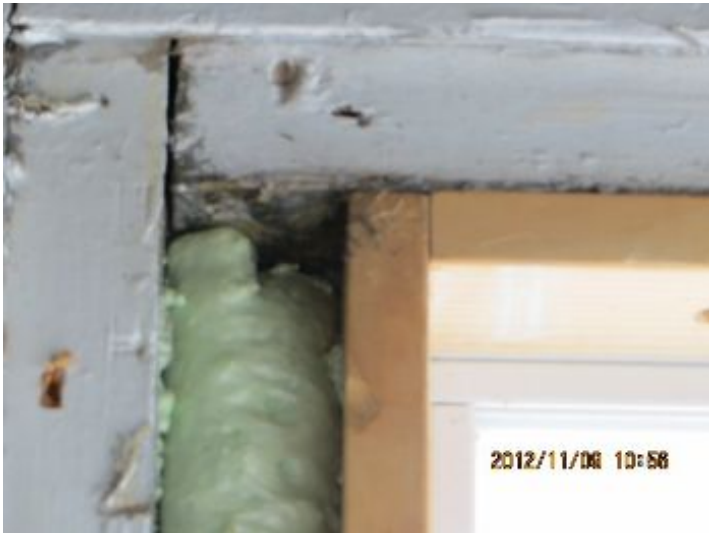
Exterior wall(s) have been cut or bored. The exterior wall is not structurally supported. Installation proper lintel is required.
