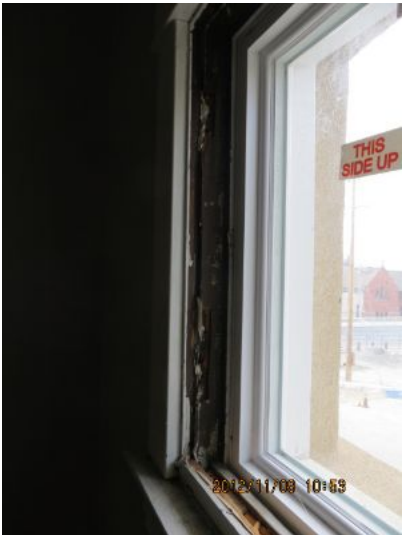
Deterioration/rot of wooden frames noted. While basic maintenance may prolong the life of these window frames, replacement may be necessary at some point.
