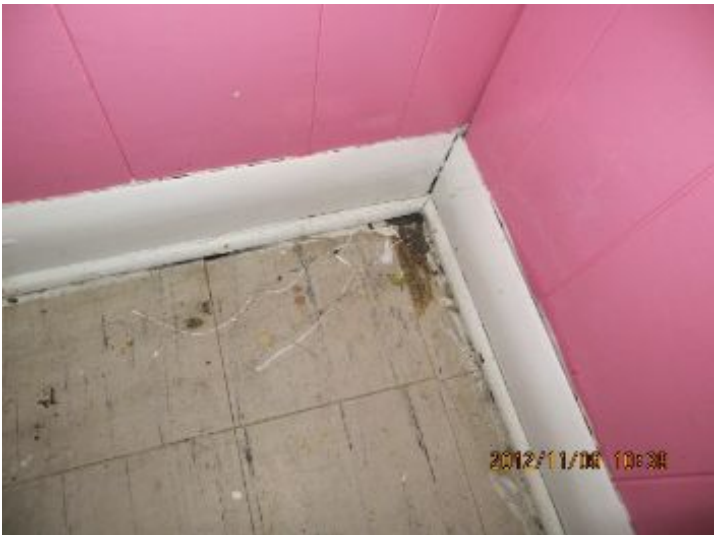
Wood rot, moisture damage observed
