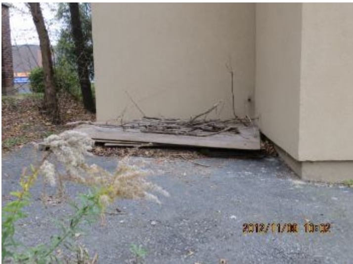
inaccessible (covered by material)At: all around
