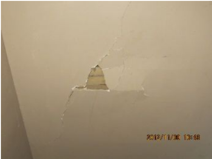
Damage(s) noted. required repair and painting.
