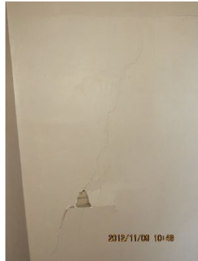
Damage(s) noted. required repair and painting.
