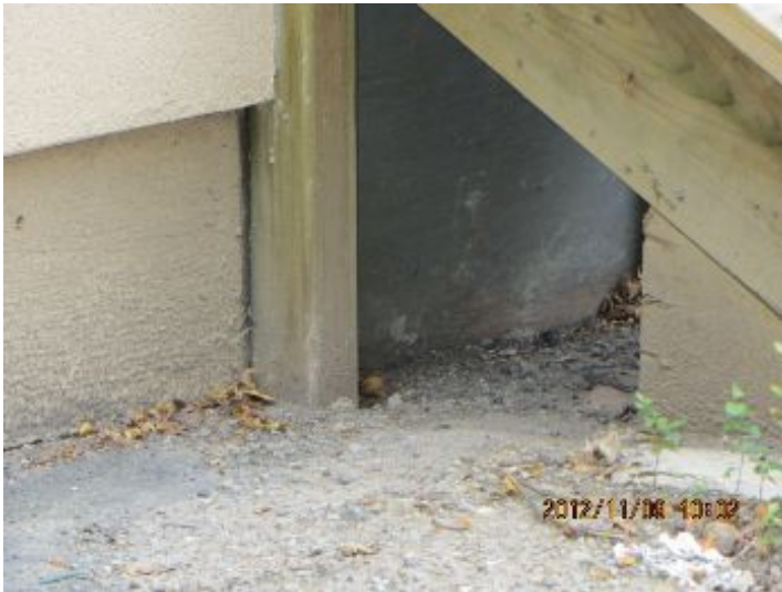
Evidence of ponding observed. At: rear
