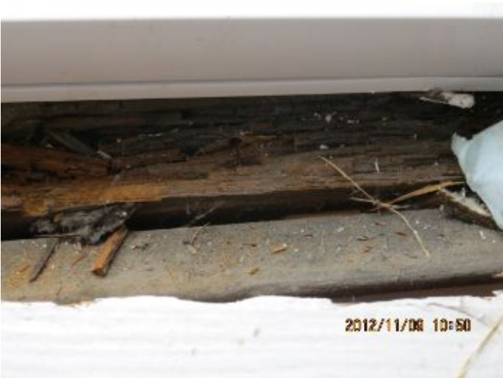
Deterioration/rot of wooden frames noted. While basic maintenance may prolong the life of these window frames, replacement may be necessary at some point.
