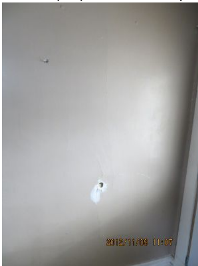
Damage(s) noted. required repair and painting.
