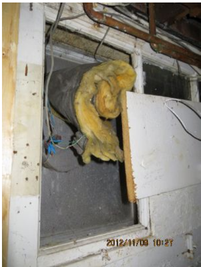
Some or all windows were blocked with materials or storage. Has to be open.
