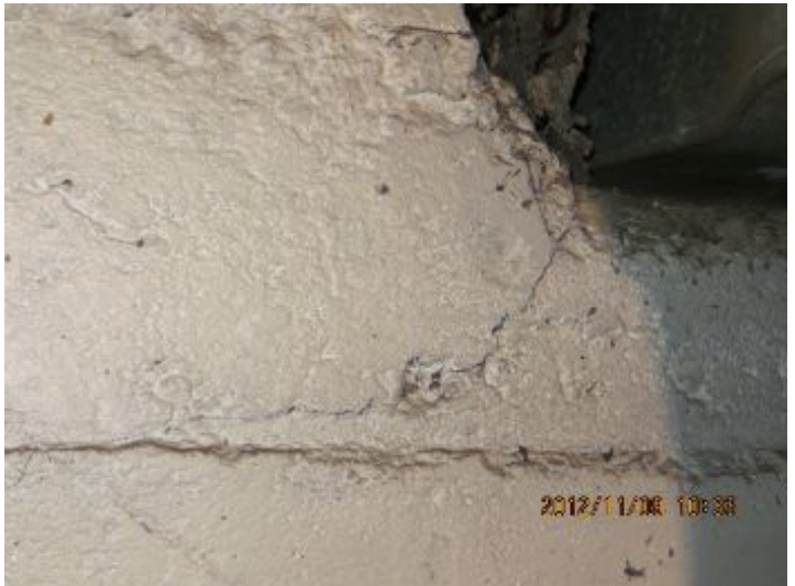
Structural crack(s) is noted. This type of crack should been assess by qualified contractor or structural engineer.
