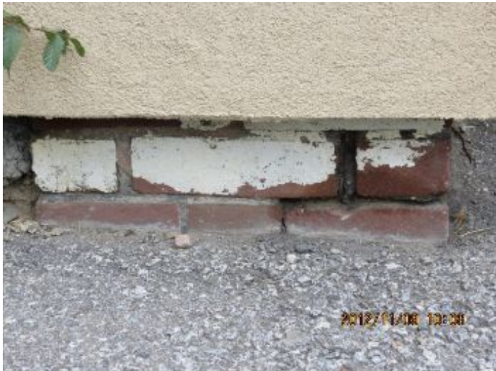
Brick to earth contact noted. This can result in water penetration & brick "spalling" or deterioration over time. Re-grading or other protection of brick is recommended. Foundation wall should extended Min 6" above finished grading. At: front
