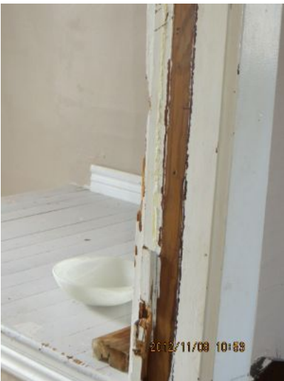
Damage(s) noted. required repair and painting.
