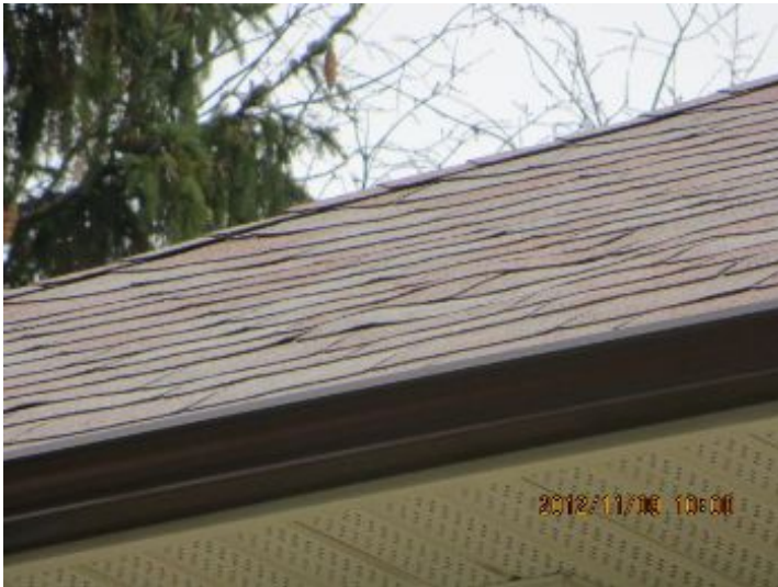
Waviness/Uneven roof surface appeared in most area of the roof. This is relatively a common condition and can be result of inadequate ventilation or water damage. At:
