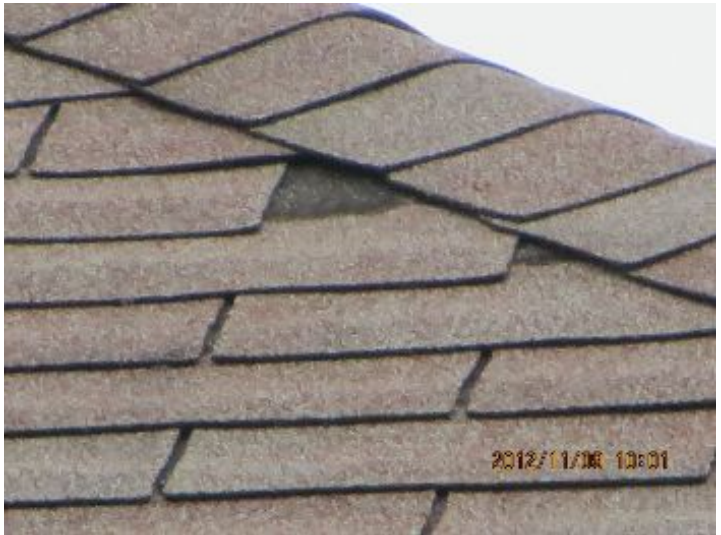
Missing shingle(s) in noted.
