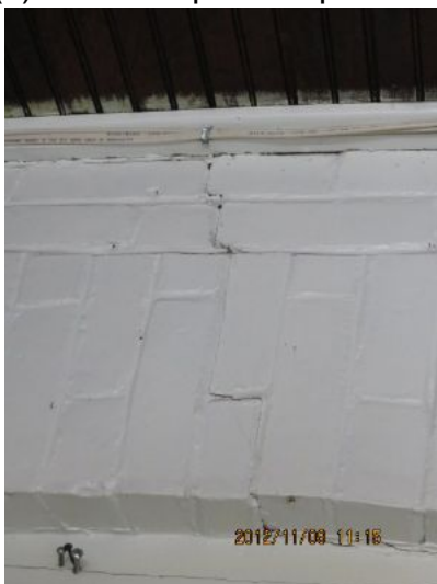
Settlement crack(s) observed. At: rear, extension part.
